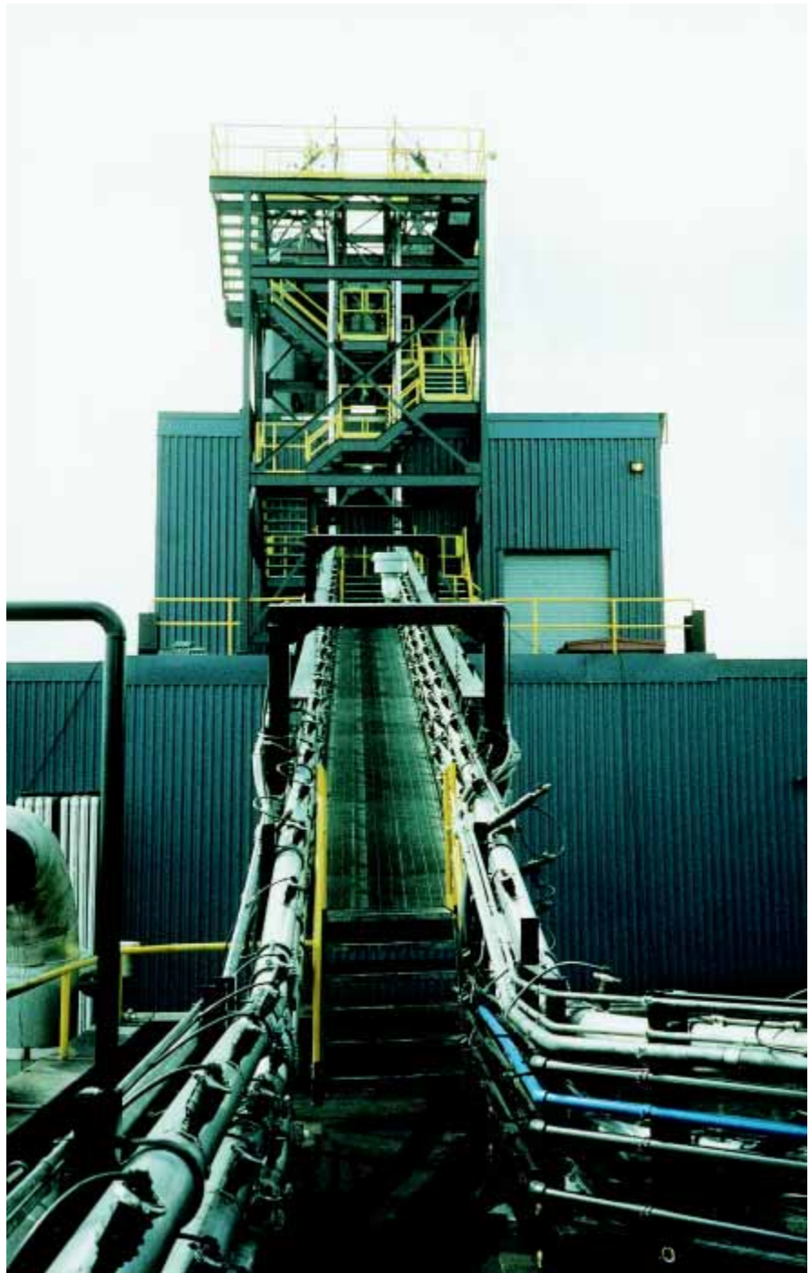
Shown above are multiple conveying lines conveying carbon black to six storage silos.
