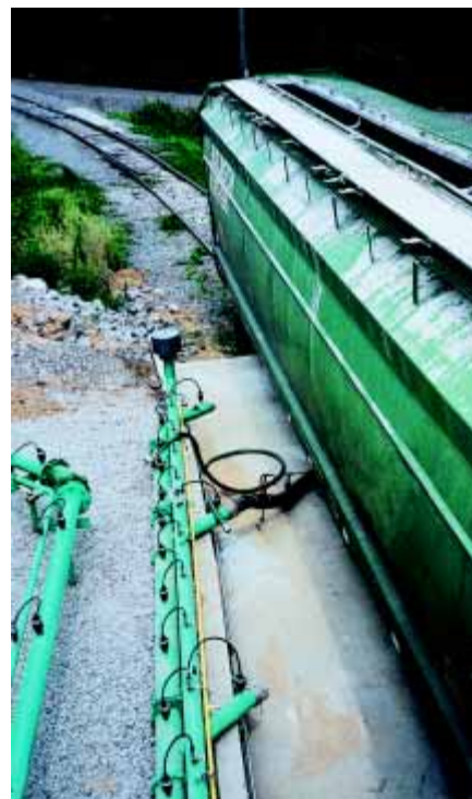
Shown above is a high density vacuum unloading system utilizing Dyna-Chek® 4 booster fittings and a vacuum hose to convey material from a hopper-bottom railcar.
