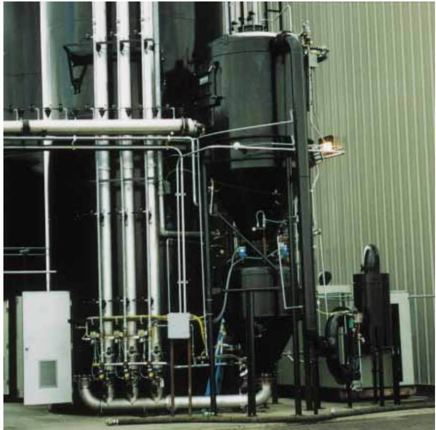
Shown above is a high density vacuum unloading system utilizing a vacuum filter/receiver mounted above a dense phase full line system to convey carbon black.
