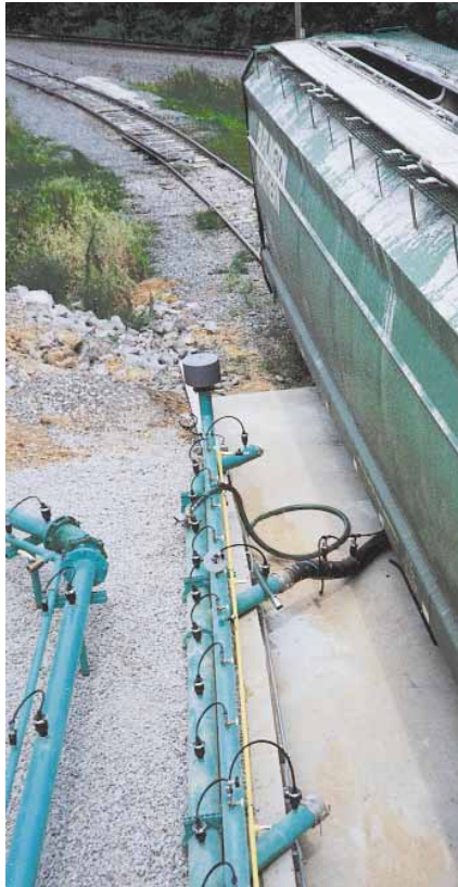
Shown above is an HDV 8000 vacuum unloading system utilizing Dyna-Chek 4 booster fittings and a vacuum hose to convey material from a hopper-bottom railcar to four storage silos.
