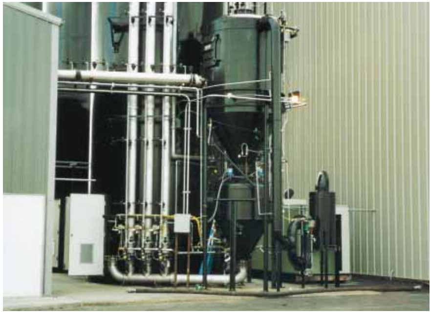
Shown above is an HDV 8000 vacuum unloading system utilizing a vacuum filter/receiver mounted above a Dense Phase Full Line system to convey carbon black from trucks to three storage silos.
