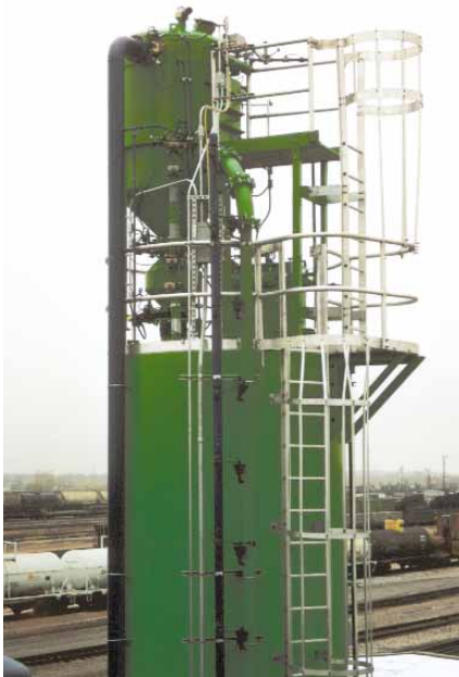
Shown above is an HDV 8000 vacuum unloading system utilizing a vacuum filter/receiver and gatelock hopper to convey sand from hopper bottom railcars to a storage silo.
