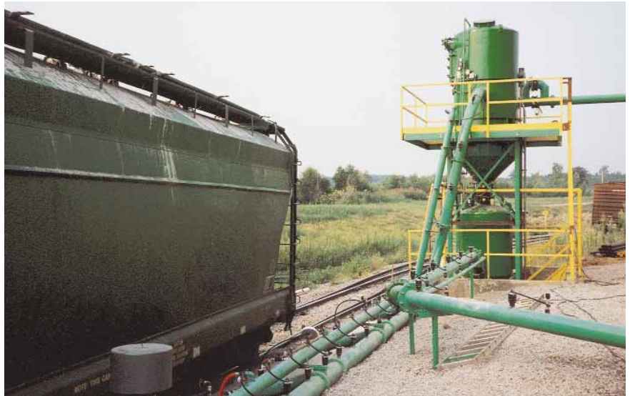
Shown above is an HDV 8000 railcar vacuum unloading system utilizing a vacuum conveying line with Dyna-Chek 4 booster fittings and a vacuum filter/receiver mounted above a dense phase pneumatic transporter.
