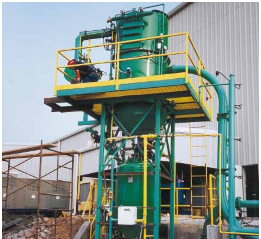
Shown above is an HDV 8000 vacuum unloading system utilizing a vacuum filter/receiver mounted above a dense phase pneumatic transporter.
