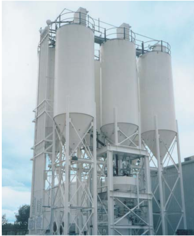
Weighing/batching and conveying system including storage silos and steel structures.
