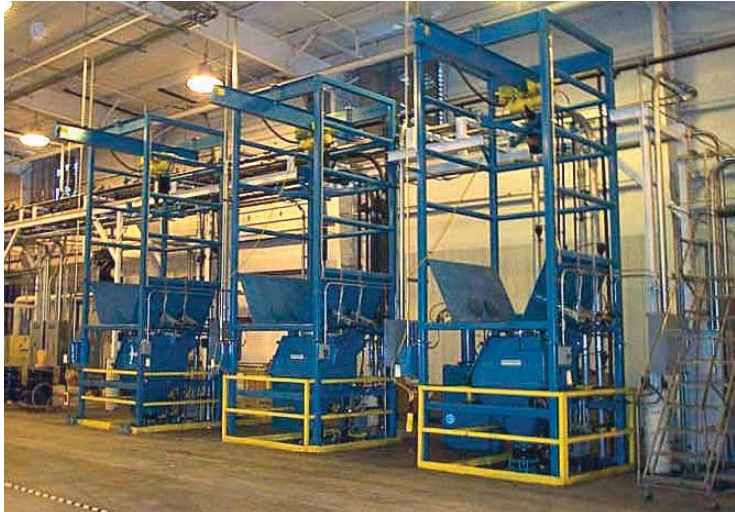
Bulk bag and small bag unloaders discharge carbon black into multiple dense phase Full Line Concept® conveying systems.
