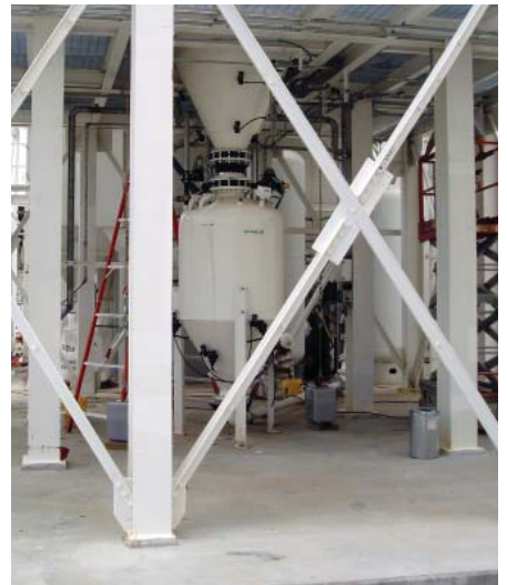
Batching & conveying systems.
