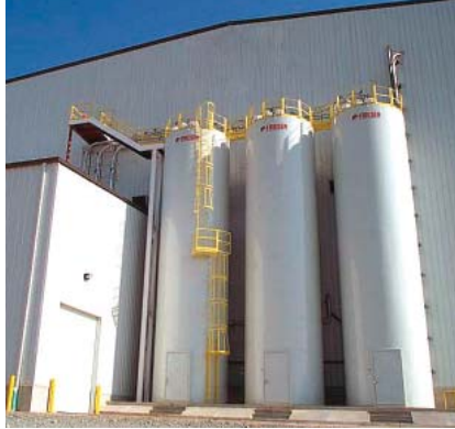
Storage silos are filled by a Full Line Concept® conveying system.
